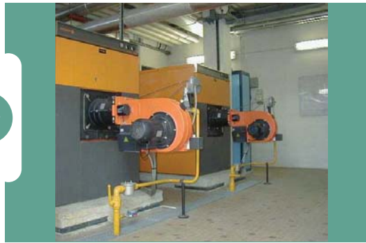
Combustion equipment (Champagne-Ardenne, eastern France)
