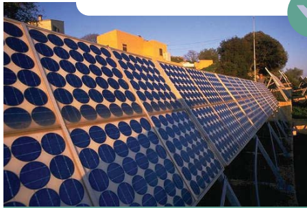
A photovoltaic generator
