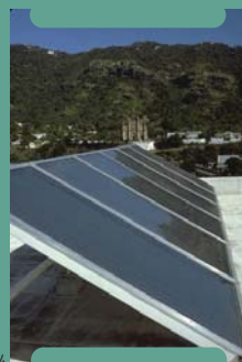
Installation powered by thermal solar energy.
