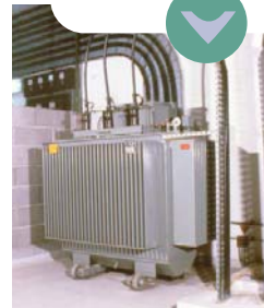
A power transformer incorporating PCB/PCTs
